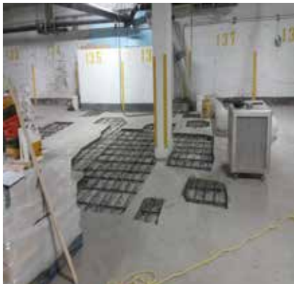
Demo of concrete degradation
